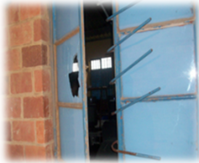
2. The window that was broken at the computer lab
